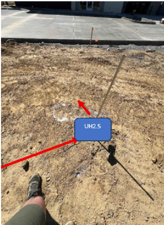
@22+66 C Spire will directional bore to the marked location flagged and white lined. CSpire will then dig down 6" and penetrate 4" conduit underground.
